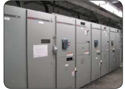
Motor Control Center Line-Up
