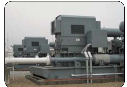
5000 HP, 900 RPM Medium Voltage Motor & Ariel Compressor Unit
